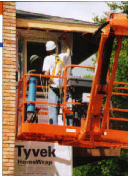
Collins Construction Co. uses its boom lift to install fascia, soffits, windows, sheeting, and more.
